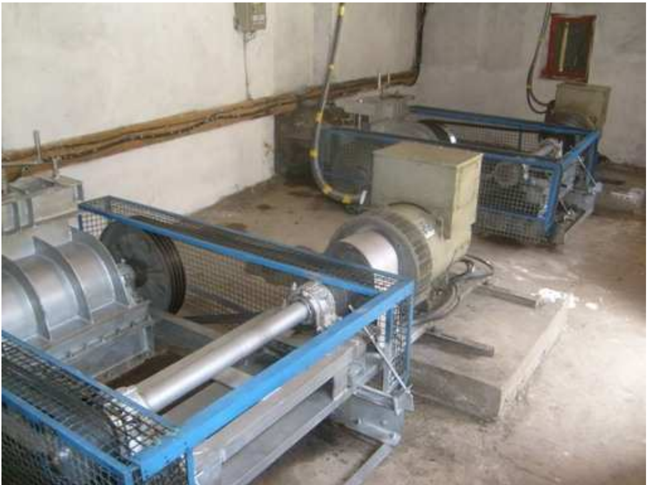
Two PT-645 turbine rated at 65kW each electrical output located at Daste Riwat, Panjshir.
